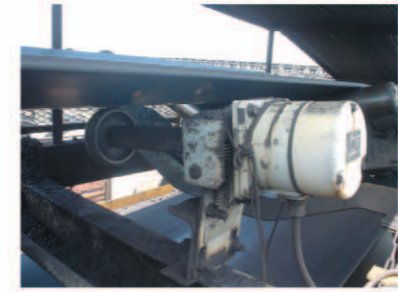
Speed Relay for conveyor slip detection
