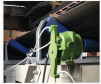
Pull Cord Switch for emergency conveyor stop
