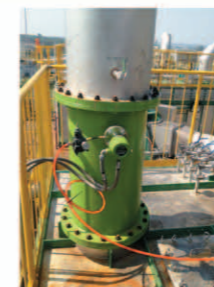
Dust Monitor for Bag filter outlet
