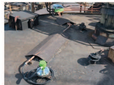
Admittance Level Switch for Upper Limit Detection for Coke hopper
