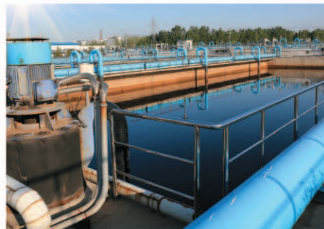
Water purification plant
