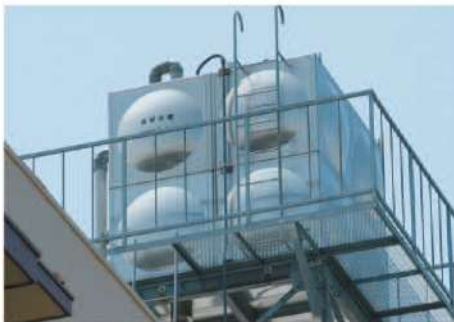
Water tank, Elevated water tank
